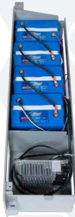
IC650 & Battery Bank
